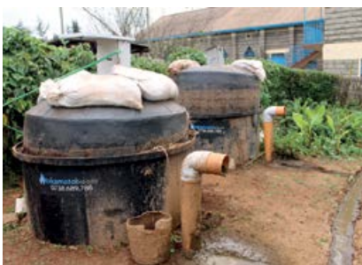
Biodigester Source: Takamoto Biogas
