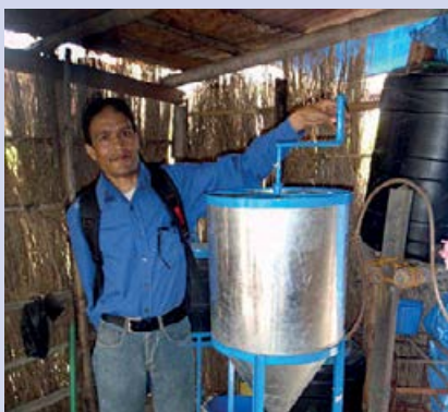
Small struvite reactor Source: Eawag
