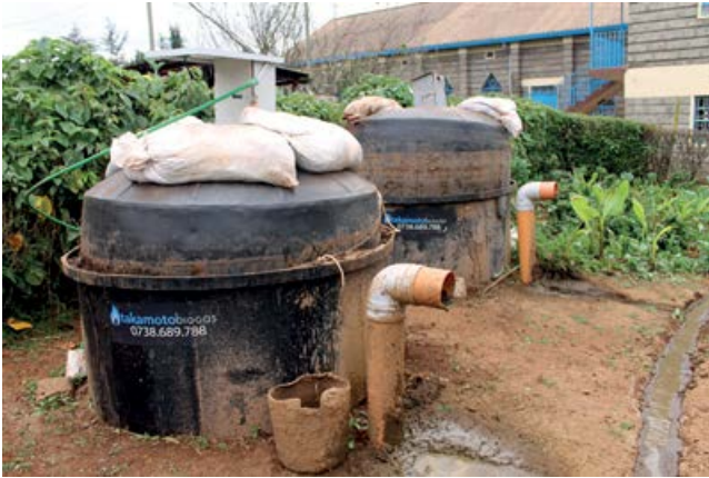
Biodigesters. Source: Takamoto Biogas
