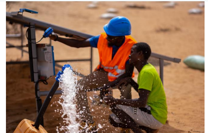
Solar pump installation, credit: Bonergie
