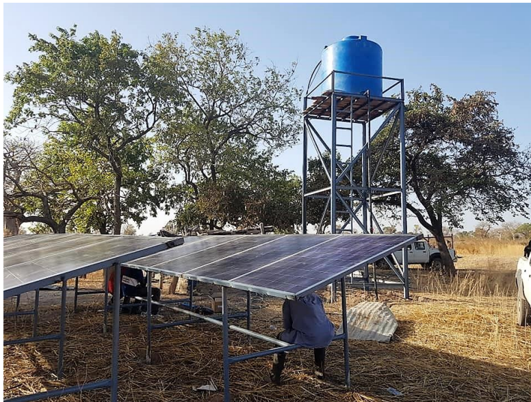
Solar pump with water tank, credit: Bonergie
