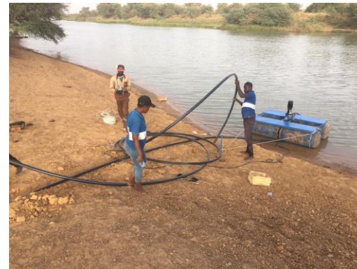
Floating solar pump on Senegal river, credit: Bonergie
